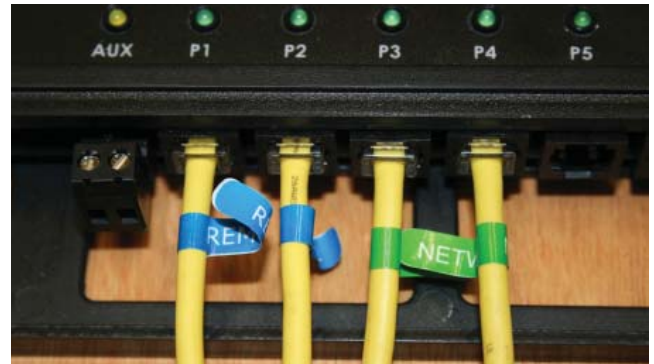
Figure 2-8, Surface Mounted Remote/Network Cables
